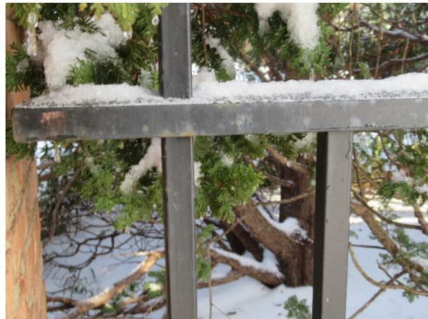
Minor fence rust
